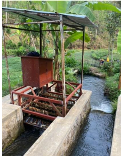
Figure 3 Pico-hydro installation on the irrigation channel at the research site.
